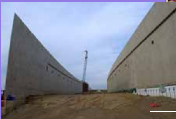
Construction of the Visitor Center continued through the spring, summer and fall of 2014.
